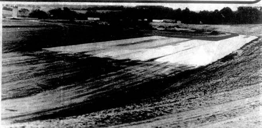
MUSHROOM PLANT CONSTRUCTION —Construction is well underway on the Ralston Purina Company mushroom plant near Loudon. The block building in the background will be the office complex of the facility. The plant itself will cover all the area graded level in the photo. The multi-
