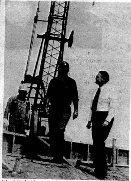
John visits site of new water treatment plant (made possible through federal funds) at Vonore—to serve major parts of Monroe and Loudon Counties.
