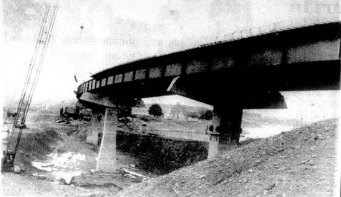
CANAL BRIDGE—Steel and concrete decking is being installed on the curved Tellico-Fort Loudoun canal bridge.
