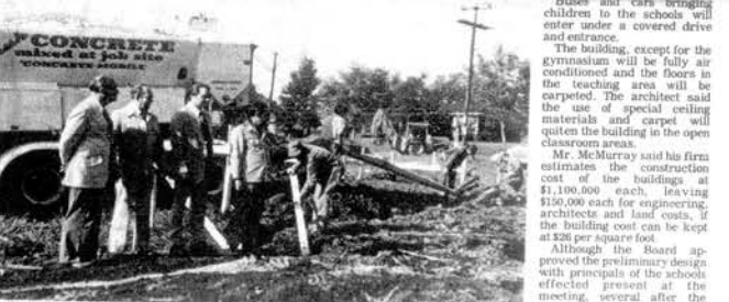
BANK CONSTRUCTION UNDERWAY—Construction began last week on the new branch of the Bank of Loudoun County on Mulberry Street in West End Loudoun near the Loudoun High School. Bank officials Ray Birkholz, Jack Randolph, President Ed Bell and Chairman J. W. Wilburn Jr. are shown as workers pour the footings for the new bank. The building is to be complete and open sometime early in 1977.
