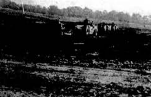
WORK UNDERWAY AT PURINA—Earthmoving equipment of Wright Brothers Construction Company has been busy for two weeks preparing the site of Purina's huge mushroom farm on Highway 72 near
