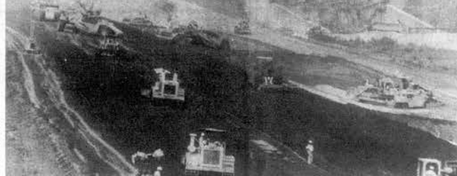
CONTINUING WORK AT TELLICO DAM - Earthmoving equipment is still spreading dirt to build the earthenfill portion of the Tellico Dam (concrete portion in background). There is still about 600,000 cubic yards of dirt to move onto the earthenfill. Work is being threatened by an injunction in federal court.
