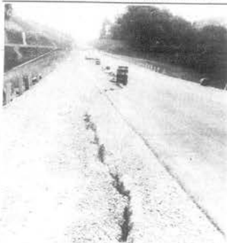
ROAD SINKS AGAIN —For the second time since it was completed last fall a section of the Sugar Linn Connector Road has cracked and sunk about a foot. Each time the damage has come during heavy rains. Engineers have said the use of improper fill material was responsible for the damage.
