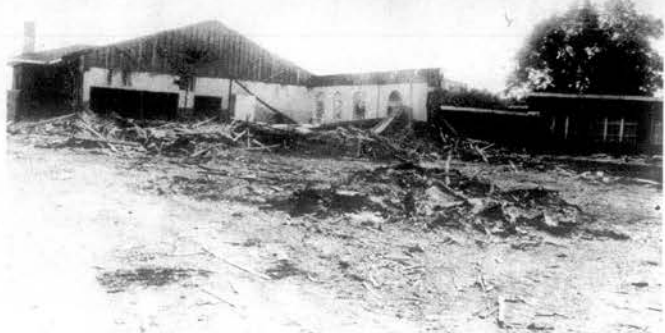
PHILADELPHIA DEMOLITION—Demolition of the auditorium is about all that is lacking at the Philadelphia school building for a new structure. The part of the building that will be kept is shown at right. When demolition is complete in mid-August it is hoped that the new $750,000 school will be ready.
