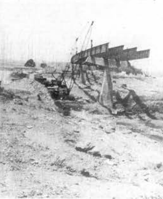
TELICO CANAL BRIDGE—Structural steel for the new Tellico-Port Loudon diversion canal is being erected
