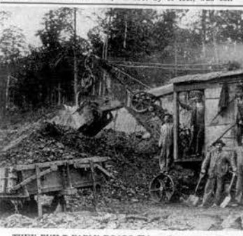
THEY BUILT EARLY ROADS—This rock quarry and crushing crew is the first county quarry after the mass introduction of the automobile.
