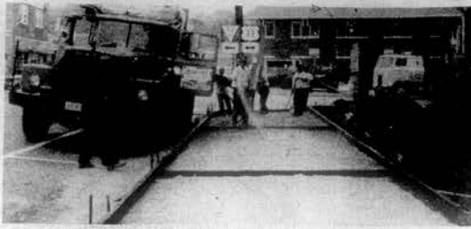
SIDEWALK REPLACED —City of Loudon street department crews are shown preparing to pour a new section of sidewalk in front of the county courthouse. The city has replaced several hundred feet of sidewalk in the area of the courthouse which has become damaged over the years.
