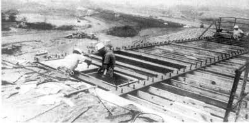
ON TOP OF TELLICO DAM—Carpenters are shown building a concrete form to allow for pouring a concrete deck over the third spillway gate of the dam. Work on the earthen portion of the dam is shown in the background.
