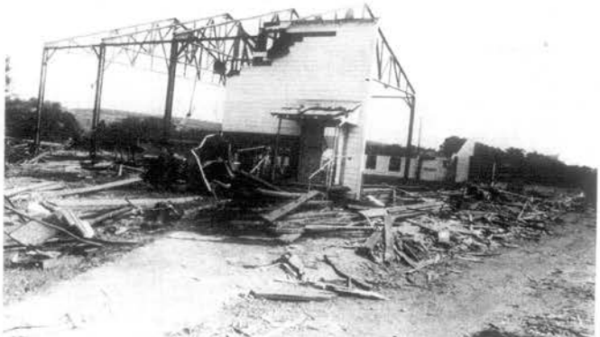
JUST A LITTLE LEFT—Only the steel frame and a little of one outside wall remained early this week of the old Philadelphia School gym as wrecking crews clear the old school building for a new structure.
