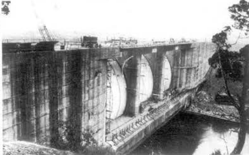
BEHIND THE DAM or upstream view of the Tellico Dam shows work going on on the dam itself. Although started almost 10 years ago the dam is still incomplete and beset with legal problems.
