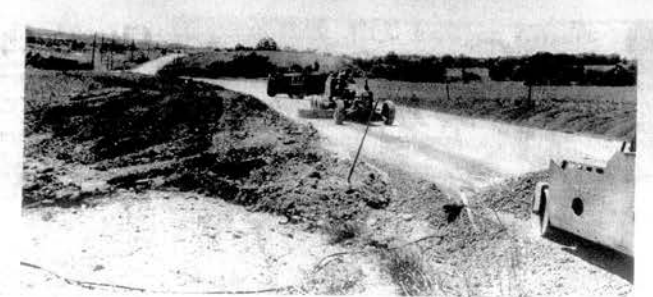
CURVE STRAIGHTENED — Loudon Street Department crews last week began a project to lessen the severity of an "S" curve in the Industrial Park Road between Highland Avenue and Maremont at Kome Street. In addition to widening the road and "sliding" the curve the road slope is being changed for more safety also.
