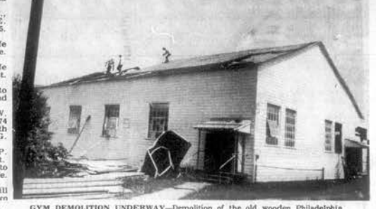
GYM DEMOLITION UNDERWAY - Demolition of the old wooden Philadelphia School gym started this week as part of a wrecking project to make the school site ready for construction of a new school. Spokesmen for Barnett Wreckers say they will have lumber and brick for sale at the site. They expect to complete their work by Aug. 15. Bids on the new school are expected about Sept. 1.
