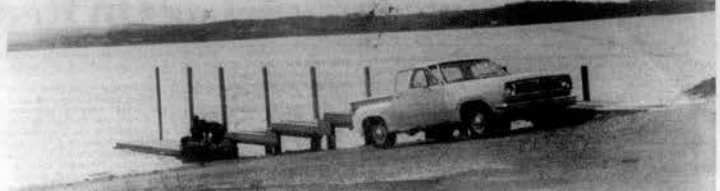
NEW DOCK TO BE COMPLETED —The new dock being constructed at the lake access ramp adjacent the Lenoir City Marina at Port Loudoun Dam will be finished this
