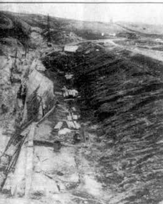
the earthfill. Construction Engineer Lamar Parker told the Herald that the job is moving smoothly. He stated there is still about 1.5 million yards of earth to be moved. About 700,000 yards have been moved at the dam site on the Little Tennessee River at this point. Spillway gates for the concrete portion of the dam are at 45 percent and the water is now pouring through the concrete portion of the dam.
