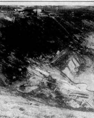
EARTHFILL FOUNDATION—Workmen on the Tellico Project, 200 of them working three eight hour shifts, continue to make progress toward the start of the filling of the lake in January of 1977. The $100 million project is to be completed at that time. In the photo above the 70 foot deep foundation for the earthfill portion of the dam is shown under construction. Once the concrete foundation is completed some 150,000 cubic yards of dirt will make up
