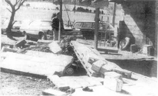
GARAGE WALL BLOWN OUT-The north wall of the garage at the Howard Bettis residence was blown out by the storm. The family's car was in the garage and was damaged when the wall collapsed.
