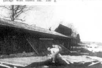
NEW RESTAURANT DAMAGED —Jim and Lou Fees, owners of the new Fees Restaurant at the Highway 72 and Interstate 75 interchange at Loudon, start cleaning up debris left in the parking lot after Sunday morning's wind storm damaged the new business that was just opening.
