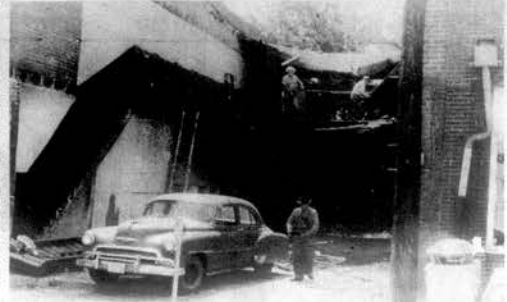
ONE OF THE OLDEST BUILDINGS in Loudon is being torn down. The building, on Grove Street, near the Legion Building, housed several grocery store operations during its more than 75 year existence. The building was condemned as unsafe by the City of Loudon last fall. The out-of-state owner decided to demolish the building rather than bring it into compliance with city commercial building codes.
