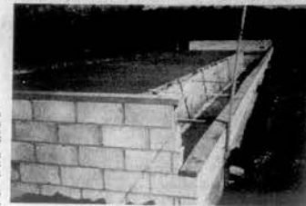
SWINE FINISHING FLOOR—Shown above in the early stage of construction is a partially slatted swine finishing floor being built on the George Miller Resource Management farm near Greenback. The building, when completed, will have ten pens that will hold thirty feeder pigs per pen for a house capacity of 300 pigs which will be topped to slaughter weight.
