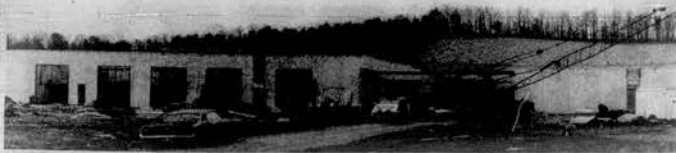
WILL OPEN IN FALL —Construction continues on the Loudon County Vocational Education Center on Harrison Road near Lenoir City. The million dollar facility is due to
