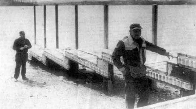
SHOWS WATER LEVEL —Mr. Robert Grindstaff of Lenoir City and Edward Brannon, both TVA employees are doing the finishing work on the new dock to be in use for this summer at the lake access ramp at the Lenoir City Marina. Mr. Grindstaff shows the expected water level that will cover the extended portion of the dock and walk
