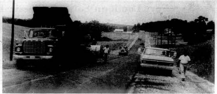
PAVING ON THE PHILADELPHIA Connector from I-75 to Highway 11 was completed Tuesday by Warren Brothers. A crew is shown putting the top coat of asphalt on the road Monday. A state engineer said that the job with shoulders, driveway entrances, guardrails and signs would be completed late this week.
