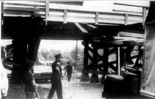
BRIDGE DAMAGED —A closed bed truck driven by James Curtis, traveling on College Avenue in Loudoun Sunday afternoon struck the overhead bridge near Loudoun Junior High School damaging both the bridge and the truck. A section of the walkway on the bridge was knocked away by the impact.
