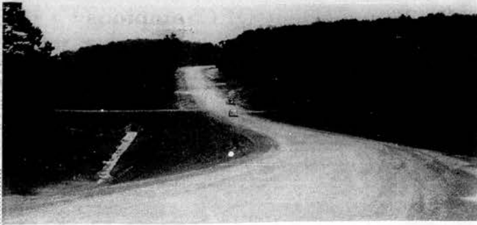
SUGAR LIMB READY FOR PAVING —Bids for the paving of the Sugar Limb connector will be opened in Nashville Friday. The roadway is nearly ready for the paving contractor as construction crews are mainly working on drainage problems at this time. The section of road pictured comes up behind the Justice Center which is about a half mile away.
