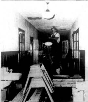
GLENDALE RENOVATION UNDERWAY-A workman is shown taking down the old lighting in a hallway at Glendale School. A $25,000 renovation project is now underway at the school to bring it to safe standards for use.
