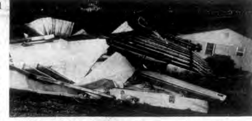
DEMOLISHED MOBILE HOME —The crumpled remains of the C. B. Watson mobile home on Loudon Hodge Road is shown shortly after it was flipped on its top during a heavy rain and wind storm Friday night. The mobile home was destroyed the family lost much of its belongings. No one was seriously injured.
