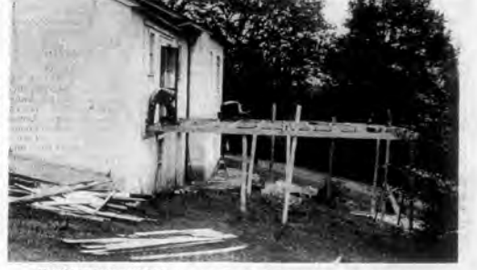
COUNTY MAINTENANCE men are shown building a sundeck on the Senior Citizens Center building, formerly the nurses quarters at Bacon Hospital. The building is being remodeled inside and out to serve as a center for senior citizen's activities.
