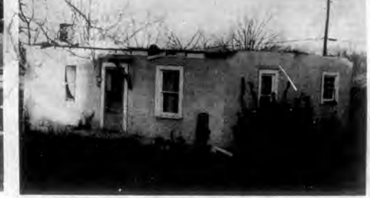
ROOF IS GONE —The entire roof structure of the Charlie Costner home on Highland Avenue in Loudon was torn off during the violent storm Friday night. The ceiling gave away allowing the heavy downpour destroy or damage most of the families furnishings.
