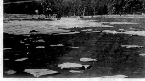
MAREMONT ROOF DAMAGE —Some of the damage to the roof of the Maremont plant in Loudon is visible in this picture. Some 30,000 square feet of roofing at the plant was damaged by the storm Friday night causing heavy damage to materials inside the plant.
