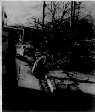
LOTS OF WORK TO DO —A South Central Bell repairman is shown at work untangling a downed line on Ward Avenue in Loudon. Many lines in the county were down by falling tree limbs such as the ones in the background.
