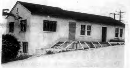
REMODELING UNDERWAY - The 1800 square foot building that will soon serve as a headquarters for Senior Citizens of Loudon County is now being remodeled through the efforts of the county, the Mid East Community Action Agency and East Tennessee Development District. The building is located next to the old Bacon Hospital.
