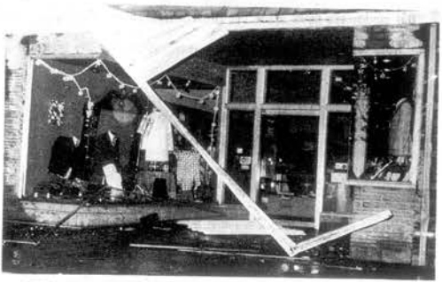
THOMAS HILLS store front was heavily damaged in the Tornado and storm as were more than 15 other businesses.
