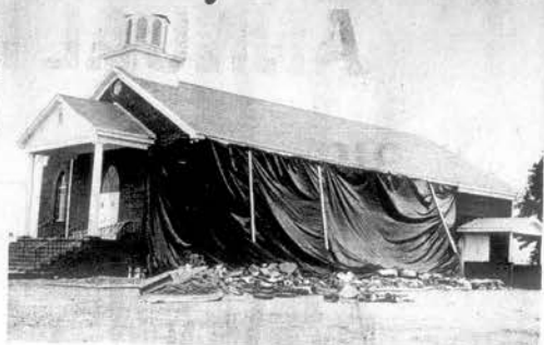
NEW PROVIDENCE DAMAGE—Sheets of black plastic over what was the west wall of New Providence Baptist Church. The wall collapsed Tuesday morning.
