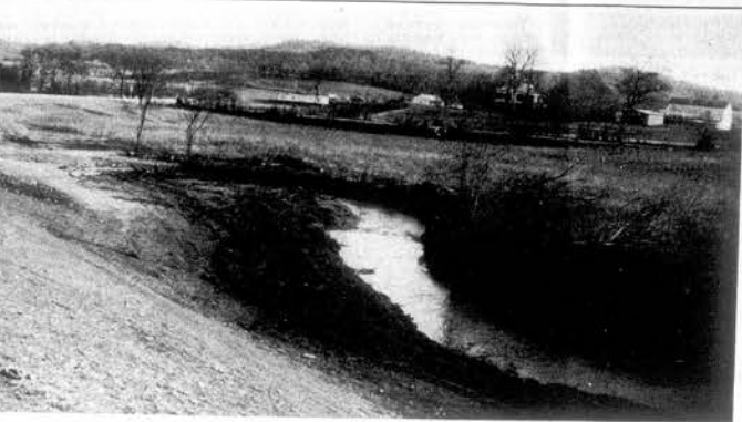
SWEETWATER CREEK WORK —Work clearing Sweetwater Creek at Philadelphia part of the multi-million dollar Sweetwater Creek Watershed project is shown underway there this week.
