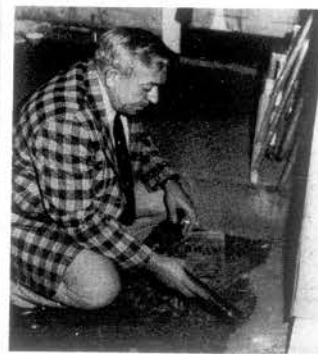
WHERE FINEST SHOT HIT—Sheriff Guy Russell examines where the first shot fired by Fred Howell to scare Kenny Dyer away from his home early Sunday struck a concrete lip on the foundation of his home.
