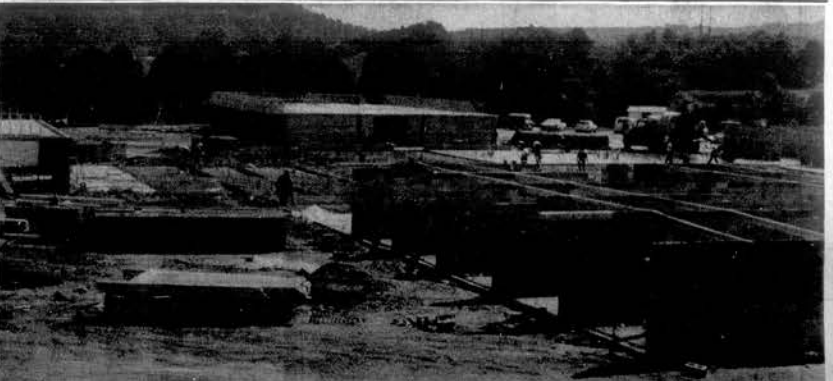
CARE INN CONSTRUCTION —Construction on several wings of the 90 bed Care Inn Nursing Home at Loudon is shown in progress. The $1 million facility is to be completed early next year. The William Bond
