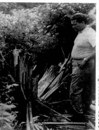
FORCE OF EXPLOSION —The force of the explosion which dented four power poles carrying transmission lines to Union Carbide can be seen in the photo. Chief Deputy Luke Bright inspects the splintered stump of what was a 90 foot power pole.
