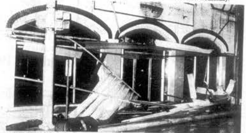
THE OLD COTTON EASTER Ford building had the aluminum front ripped off in the tornado.
