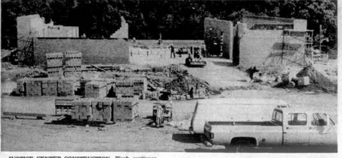
JUSTICE CENTER CONSTRUCTION —Work continues on schedule on the $700,000 Loudon County Justice Center complex on U.S. 11 between Loudon and Lenoir City. The Center, which will house a county wide communications
