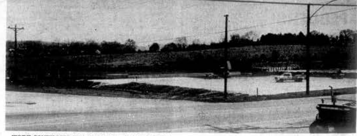
WORK CONTINUES ON LOUDON CITY RECREATION PARK —The Loudon City Recreation Park continues to bloom with spring. The 11 acre $290,000 project completed the swimming pool last summer and contractors are busy putting the finishing touches to two tennis courts on the east and west sides of the pool area. A multi-purpose court
