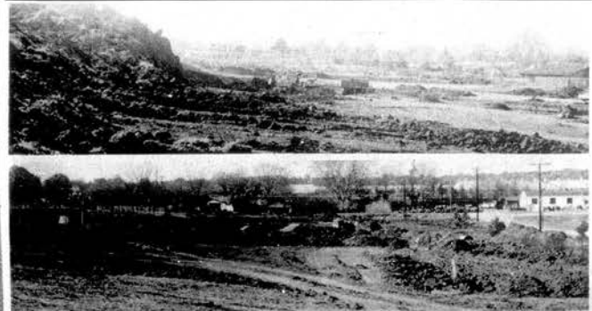
LOUDON PARK CONSTRUCTION—Construction is well underway on the second phase of development at the $200,000 City of Loudon Recreational Park. Swimming Pool complex. The movement of dirt in the area of the tennis courts has been completed and construction on the
