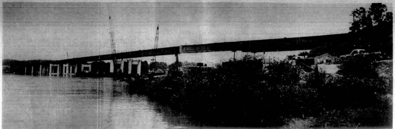
STEEL FROM BANK TO BANK—Steel erection crews last week put in place a 90 foot section of steel that linked the I-75 bridge on the Tennessee River from bank to bank.
