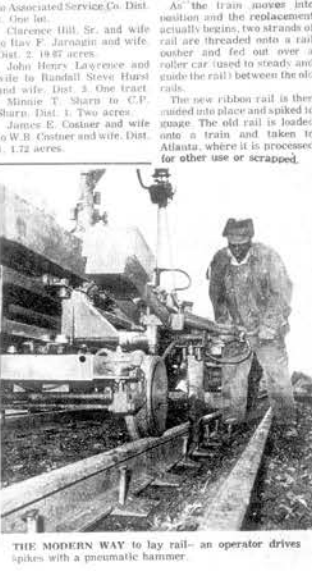
THE MODERN WAY to lay rail—an operator drives spikes with a pneumatic hammer.
