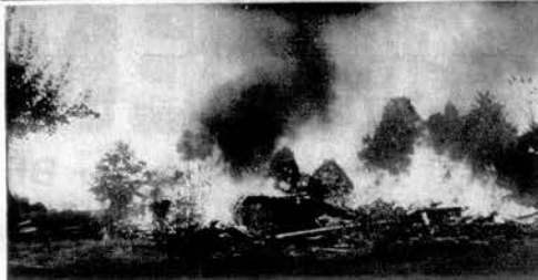
AN OLD HOUSE at Riverside Cemetery in Loudon which was being torn down caught fire and burned Friday afternoon. Loudon Fire Chief Chili Jones said since the house was being demolished it was allowed to burn, but the fire department equipment and men stood by to prevent the fire from spreading to other nearby residences.
