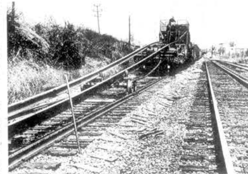
WELDED RAIL ROLLS off specially designed cars that carry it into the track bed where it will be replaced with standard jointed rails already there.
