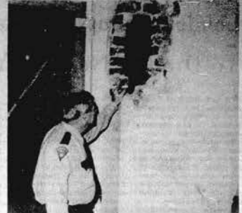
ESCAPE BID - Loudon County Deputy Guy Russell looks at a hole in a chimney wall in the drunk tank area of the Loudon Jail where two inmates, the only ones in jail at the time, are charged with attempting to break out of jail by digging through the brick walls.
