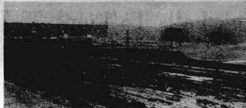
POOL CONSTRUCTION STARTED —Although now halted by rain construction did start last week on the new Olympic swimming pool in Loudon next to Loudon High School. The $74,000 pool, part of an overall $280,000 park development will be ready for use next spring.
