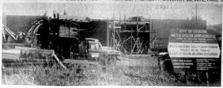
90 DAYS FROM COMPLETION - The new two million gallon per day water treatment plant for the City of Loudon, located on the Tennessee River, is expected to be completed in April. Utility Manager Charles Burnette
