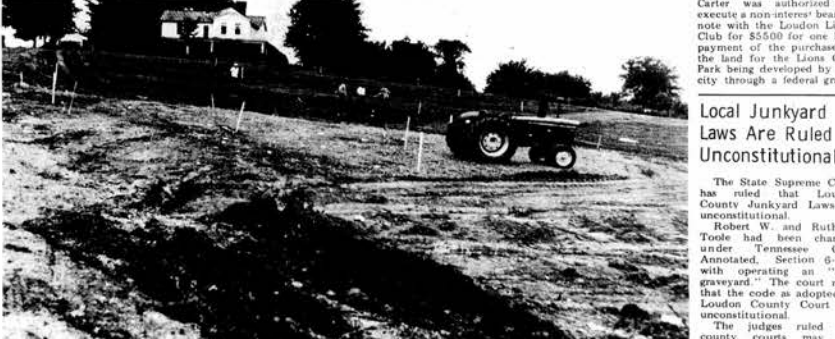
HOUSING PROJECT WORK UNDERWAY-A crew of workmen are shown staking out the 60 units of the million dollar Loudon Low Rent Housing Project which is now under construction on an 11 acre site on the old Duff farm overlooking the Tennessee River at Loudon. Excavation on the site is to be completed in three weeks.
