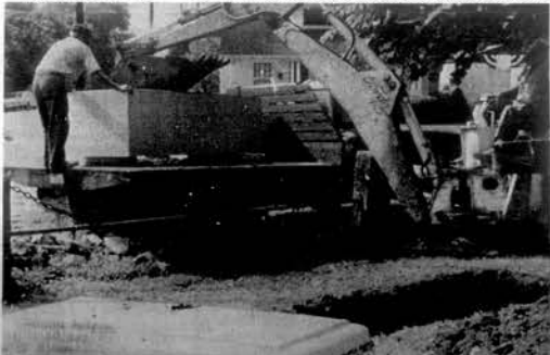
TIME CAPSULE SITE PREPARED—Workmen are shown preparing to place a concrete and steel vault in the place prepared early this week for the burial of the Loudon County Centennial Time Capsule. The capsule, to be buried in the courthouse lawn, at the site of the old hitching rack, has room for 1000 Loudon Countians to place items in special envelopes, that cost $1 each. The capsule burial is set for 12 noon Saturday. It will be opened in 50 years.
