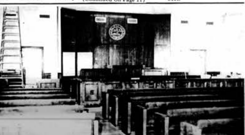
COURTROOM ALMOST READY—Work on the main courtroom at the Courthouse in Loudon is almost complete. For about two months the courtroom and other areas of the courthouse have been undergoing some $55,000 worth of remodeling. In the photo above the courtroom with a new judges bench and new furniture throughout is shown. Another smaller in size due to the addition of a jury room, meeting rooms, another rest room the new courtroom will feature air conditioning, lower ceilings, better lighting and will be sound proof. Work on the courtroom is scheduled to be completed this month.
