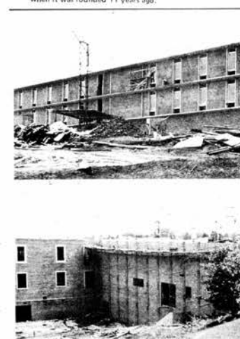
HOSPITAL TAKING SHAPE—These two photos (the top one showing the front view) show the progress being made on the new $2,000,000 Loudon County Memorial Hospital which is scheduled to open late this year. The bottom photo shows the rear area (service area) of the 50-bed major surgical and medical facility being built immediately behind Bacon Hospital in Loudon.
