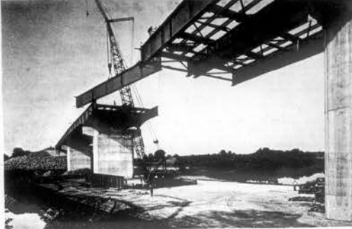
STEEL GOING UP —As part of its Tellico Reservoir project, TVA is completing steel erection for a major new bridge that will carry U.S. Highway 411 over the new lake near Vonore. The four-lane bridge will be 1,000 feet long, and will require 2,200 tons of steel.
