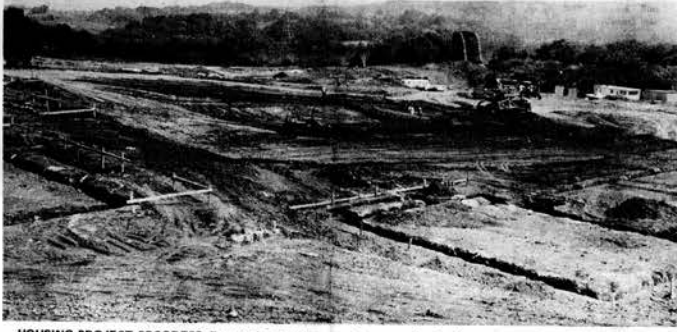
HOUSING PROJECT PROGRESS—Progress in preparing the 12 acre site of the 50 unit Loudoun Low Rent Housing Project is shown in the above photo. Some of the footings for the duplex units are shown in the foreground and others are scattered over the acreage to a point near the railroad bridge in the background. The million dollar project is expected to be completed late next year.
