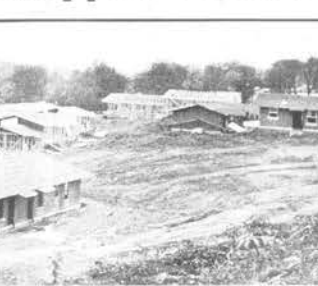
The million dollar project, financed with federal funds, is scheduled for completion in June of 1971. The project is located on Fort Hill in Loudon overlooking the Tennessee River on the old Duff farm.
