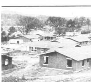
HOUSING PROJECT CONSTRUCTION—Work on the construction of 50 low rent housing units in Loudon is continuing on schedule. Above some of the units, mostly duplexes, are shown in various stages of construction.
