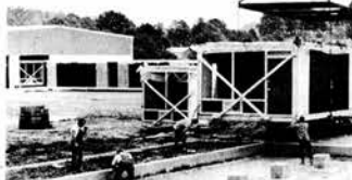
MOTEL ROOMS CONSTRUCTED—A large crane at Lenoir Industries, Highway 95 and 175, Lenoir City, moves a pre-fabricated motel room into place. A final unit then will be finished on top of the first to complete the eight room unit. Workers then add finishing touches on the outside of the building.
