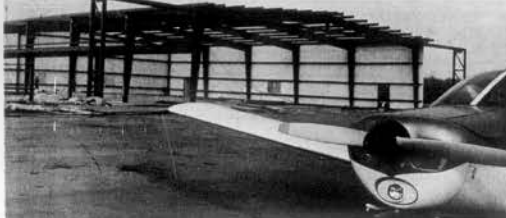
NEW HANGER AT MONROE AIRPORT —Workmen are shown applying the metal siding on the new hanger at Monroe County Airport. The 100 by 165 foot building is expected to be completed by late December or early January. In addition to providing hanger space for the 15 planes now based at the airport the building will also house office and workable facilities for the airport.
