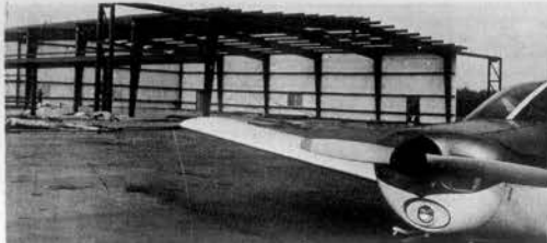
NEW HANGER AT MONROE AIRPORT —Workmen are shown applying the metal siding on the new hanger at Monroe County Airport. The 100 by 165 foot building is expected to be completed by late December or early January. In addition to providing hanger space for the 15 planes now based at the airport the building will also house office and workable facilities for the airport.
