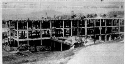
HOSPITAL CONSTRUCTION CONTINUES—The new Loudon County Memorial Hospital, a $2,000,000 project, is pictured as workmen complete the concrete work on the top level of the three floor, 50 bed hospital. Construction is expected to be completed late this year or early in 1971. The new hospital is located behind the present Bacon Hospital in Loudon.
