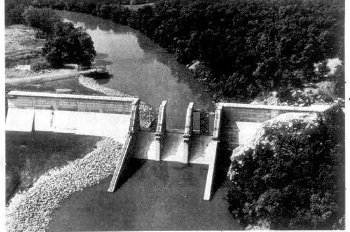
TELLICO DAM now being built by TVA is near the mouth of the Little Tennessee River in Loudoun County.
