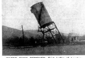
WATER TANK REMOVED—Fred Lefler of Loudon assisted in the removal of this old steam engine water tank which was done to make way for the modern diesel engines.
