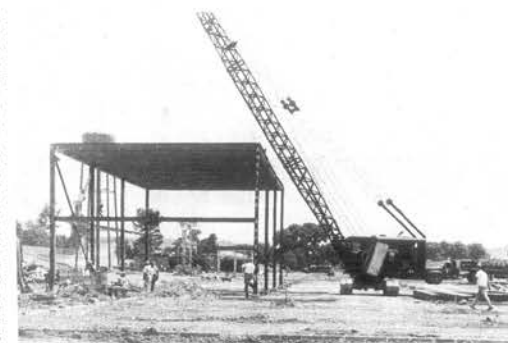
CONSTRUCTION BEGINS-In June of 1956, construction began on the 180,000 square foot Loudon plant of Union Carbide located on the banks of the Tennessee River.
