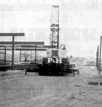
GENESCO STEEL GOING UP —Workers this week started erecting steel for the new GENESCO (Charles H. Bacon) Hosiery plant in the Fort Loudon Industrial Park at Loudon. The building, some 260 feet by 300 feet in size, will house the shipping and finishing departments of the plant which now has two other plants in Lenoir City and Loudon. The expansion project is expected to cost about $1,800,000 and will employ about 300 persons.
