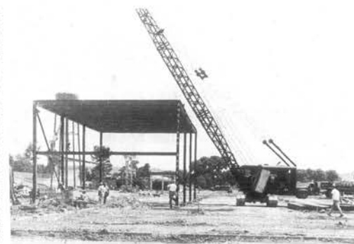
CONSTRUCTION BEGINS-In June of 1956, construction began on the 180,000 square foot Loudon plant of Union Carbide located on the banks of the Tennessee River.
